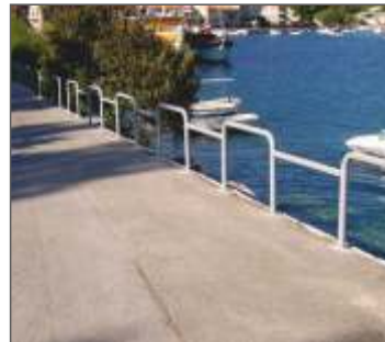
TIP 7420 - Protective fence
